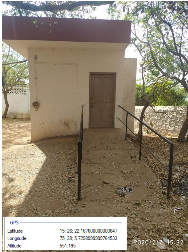
Figure 1 Disabled Friendly Washroom
